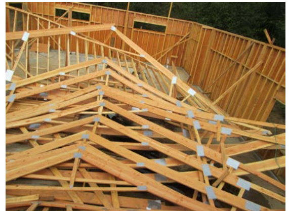
Figure 1. Collapsed trusses where the incident occurred.
