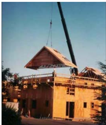
Example 1. Erecting and sheathing a series of trusses on the ground and then lifting the unit into place with a crane.
