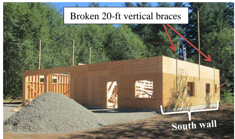
Figure 2. The shop/garage building with collapsed trusses within the structure. Note the 2X4's nailed to the outside of the south wall and that ground bracing was not erected. Middle vertical brace remained unbroken.
